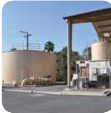
Lester Treatment Plant
